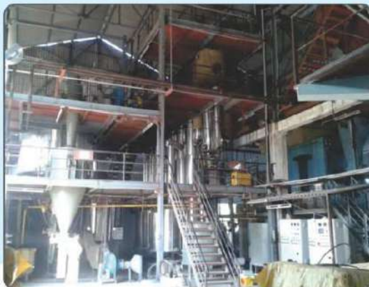
Evaporator and Spray Dryer
